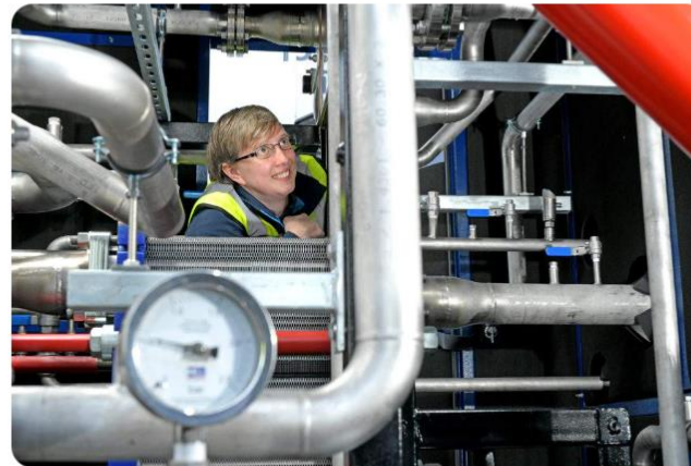
Hepworth Brewery's new type of heat pump provided by Futraheat. Photo: Futraheat Contact: Neil Davidson - neil@neildavidson.org PR Handout - Free to use
